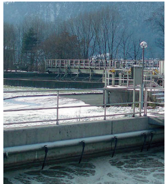
Modern large-scale sewage treatment plant: Strass sewage treatment plant in Austria
