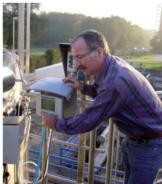
Fig. 2: Mr. Faust from the Hanau waste water treatment plant (Germany) working with an IQ SENSOR NET system and the described VARiON® sensor
