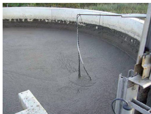
Fig. 1: Use of the VARiON® sensor in the SB reactor of the Hanau waste water treatment plant (Germany)
