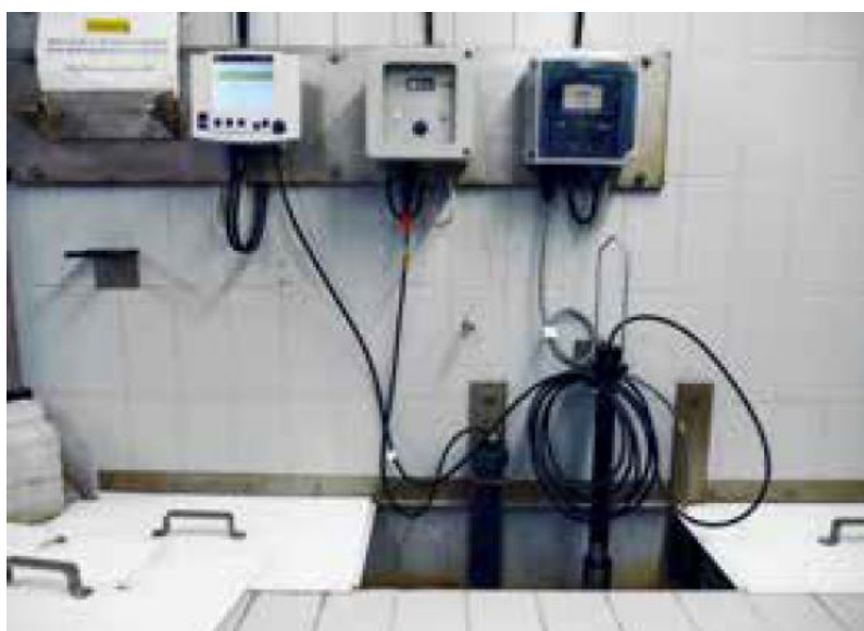
Installation of the spectral sensors (bottom right) with the controller MIQ/TC 2020 XT (top left).
