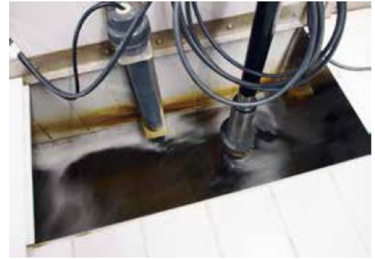
Wastewater treatment plant Regensburg - TOC measurement in the drain
