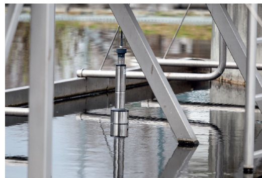
Figure 2: Typical location of the IFL 700 IQ on a scraper bridge in the secondary clarifier
